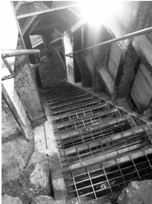
Figure 3: Steps communicating between the exposed “Herodian Street level” and the drainage system located at a higher level. Photo by K. Galor.
