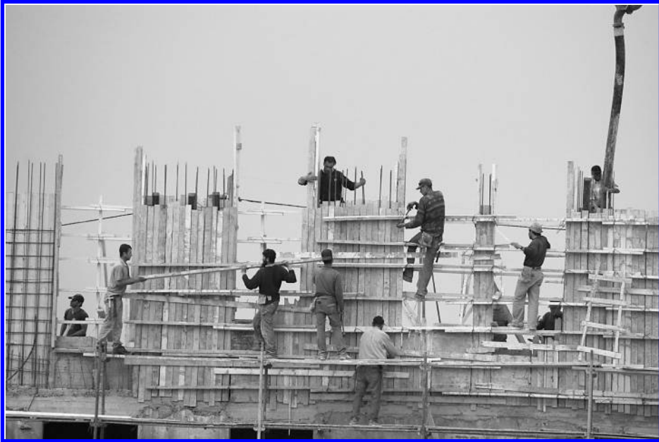
Palestinian workers construct new housing units in the Givat Ze'ev settlement near Jerusalem, 10 March 2008. (Yehuda Raizner/AFP/Getty Images)
