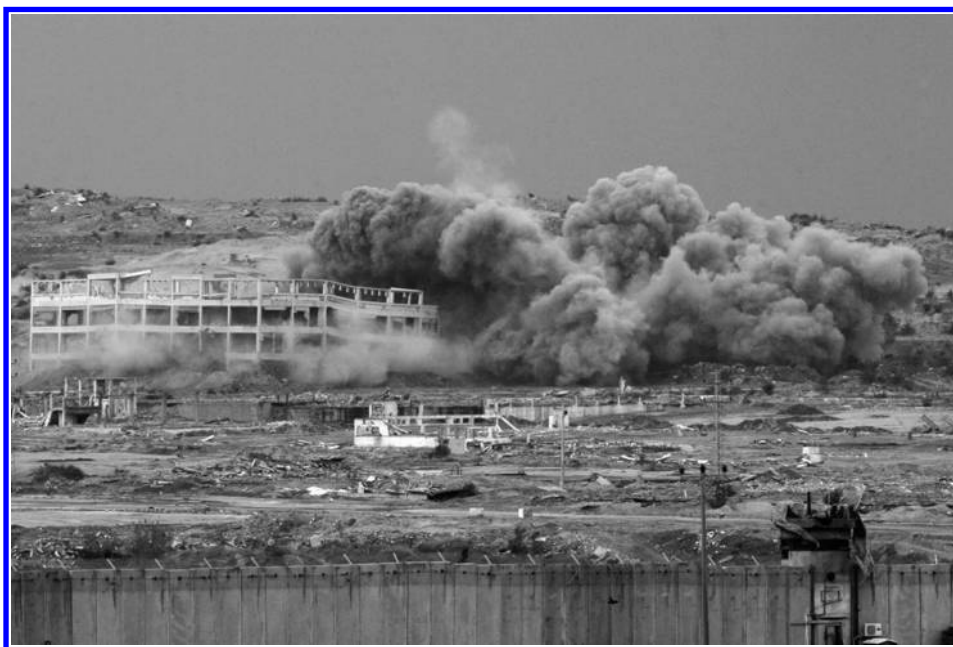
A controlled explosion takes down a building in the former Erez industrial zone, where the Israeli army leveled land to create a buffer zone and staging area for incursions into Gaza, 14 February 2008. (Menahem Kahana/AFP/Getty Images)
